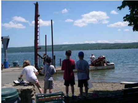
Chloe, John, William, and Noah watch the piles being driven for the new swimming dock.
